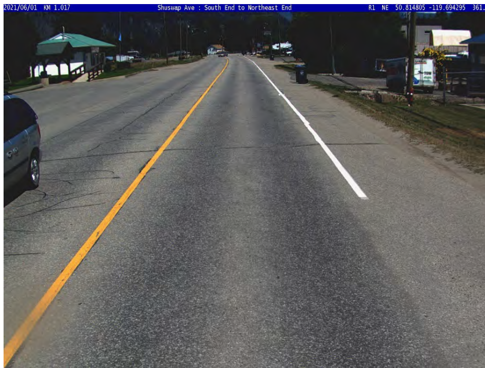
Figure 7 - High Severity Rut- Segment located on Shuswap Ave (from Brooke Dr to Mason St)
